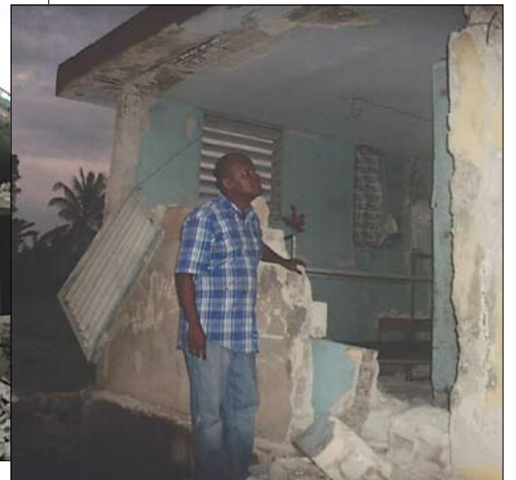
The Rev. Ron Joseph looks into the collapsed building that was the four-story orphanage before the earthquake struck Leogane, Haiti, Jan. 12.
